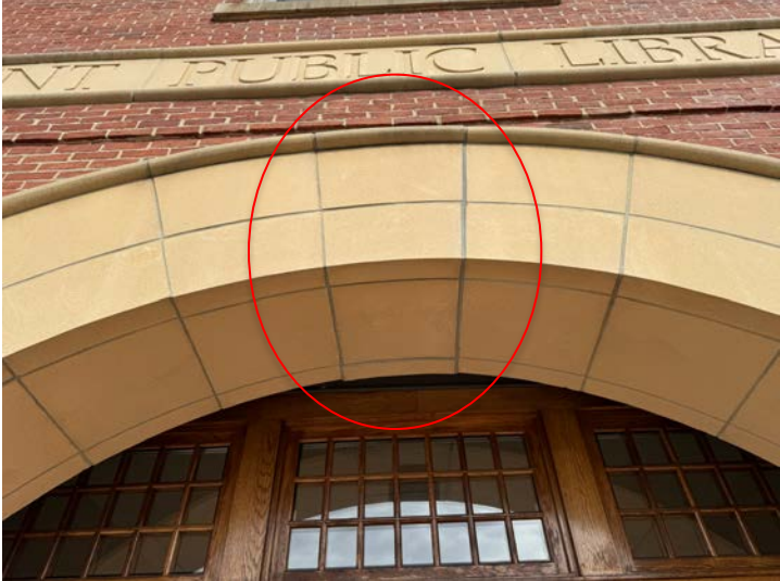
Fig. 29. Open mortar joints in arch.
