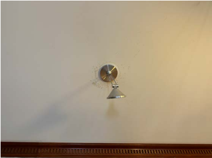
Fig. 17. Water staining around light fixtures in balcony.
