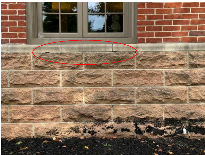
Fig. 28. Open mortar joints at the belt course and base.
