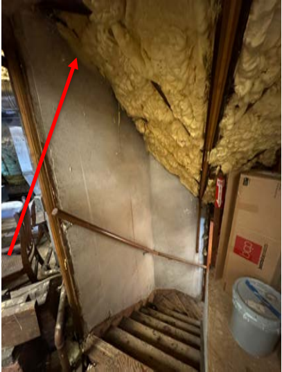
Fig. 20. Location of water infiltration.
