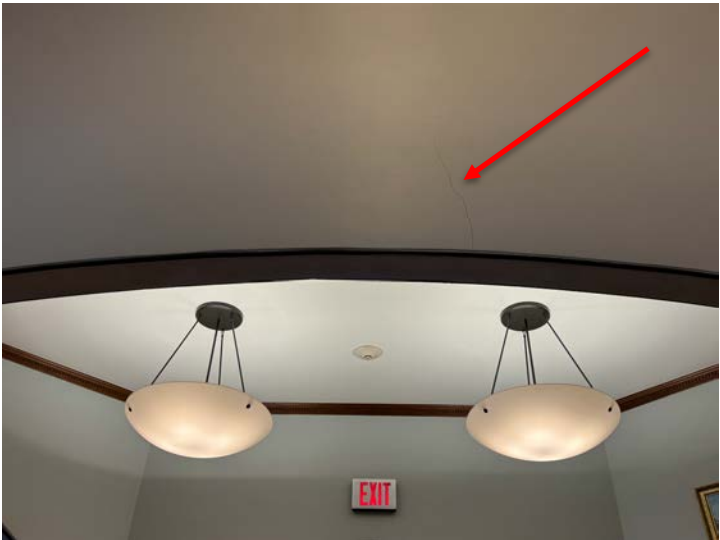
Fig. 19. Small crack in plaster over arch.
