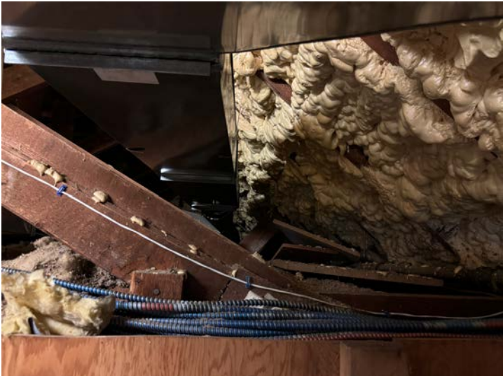
Fig. 23. Attic area above balcony light fixtures, inaccessible for leak investigation.
