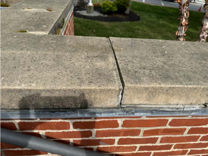
Fig. 34. Gaps at joints between shifting capstones.
