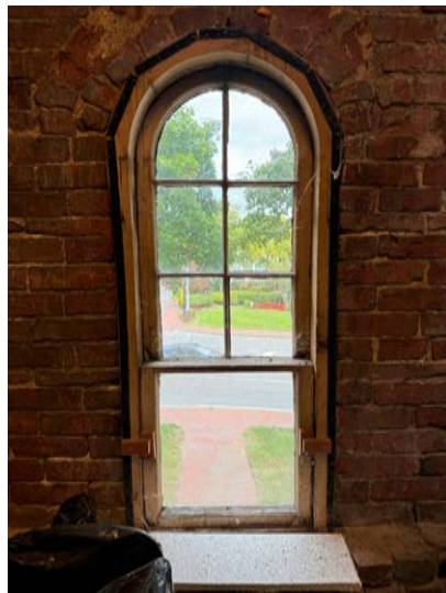
Fig. 14. Double hung wood window in attic in poor condition.
