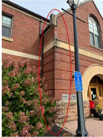
Fig. 26. Dark soiling from gable runoff.
