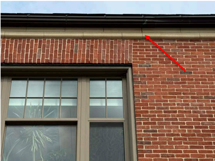
Fig. 30. Isolated cracks in cast stone.
