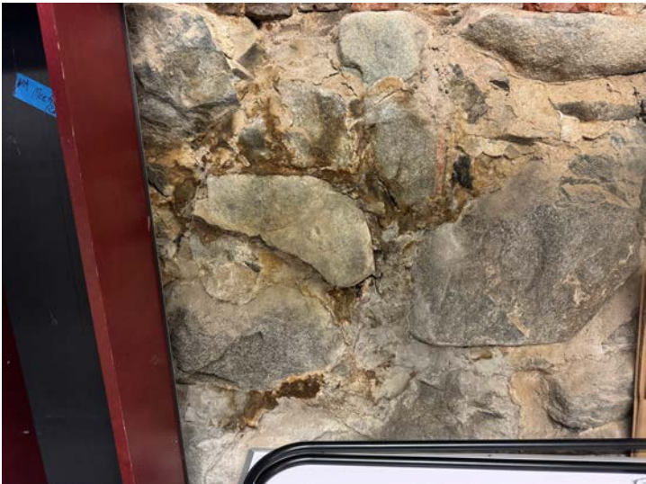
Fig. 25. Dark staining at mortar joints, possible mineral leaching from soil.
