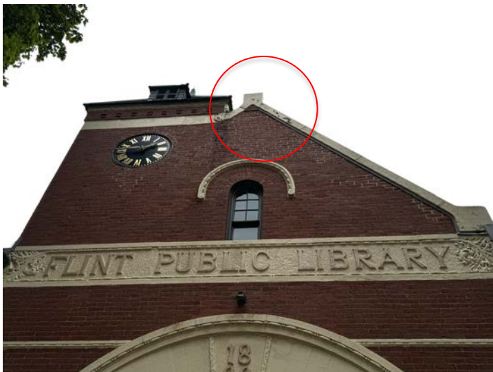
Fig. 3. Paint coating peeling from sandstone trim at gable.
