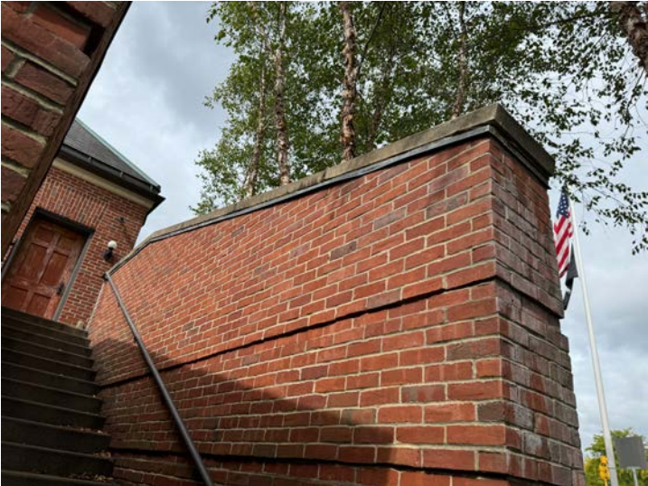
Fig. 33. Capstones at east stairs are shifting.
