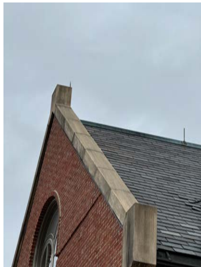
Fig. 27. Cast stone gable with through wall flashing between cast stone and brick.
