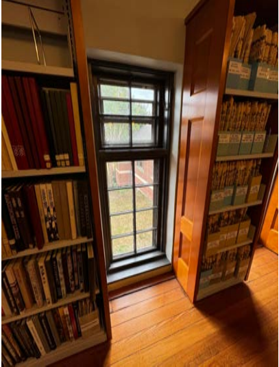
Fig. 18. Wide gap between floor boards along east and west walls in balcony.
