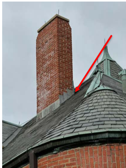
Fig. 2. Flashing around southeast chimney could be causing leaks below.
