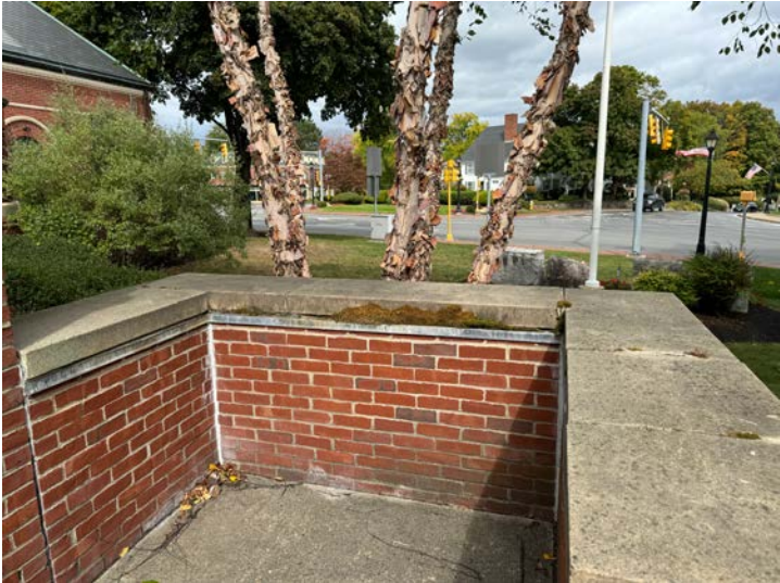
Fig. 35. Biological growth at stair capstone joints.
