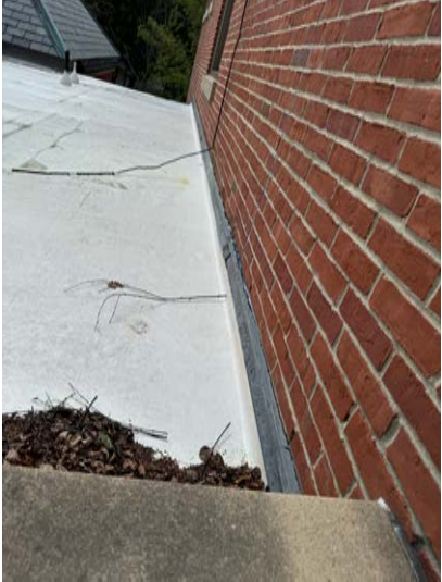
Fig. 38. Defective flashing above water leaks in Children's Library ceiling tile.
