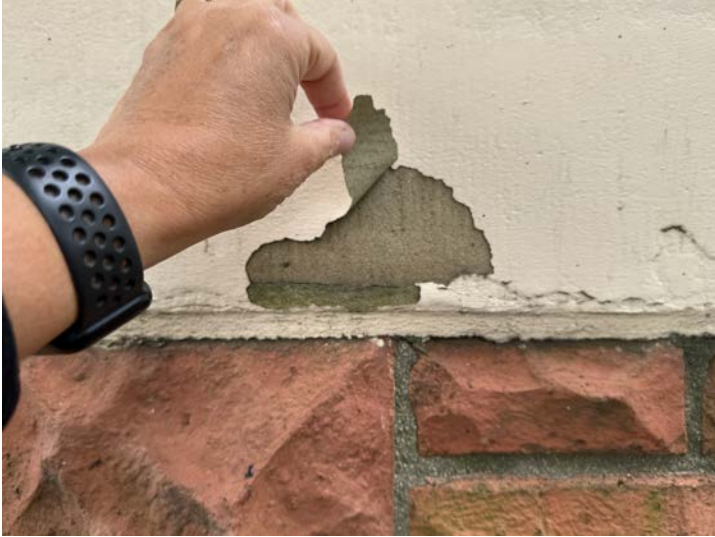
Fig. 4. Paint peeling from sandstone trim at beltcourse.
