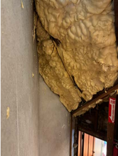
Fig. 21. Location of water infiltration at attic stairs.
