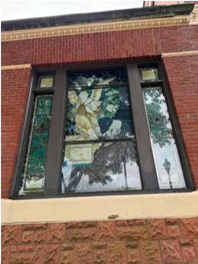
Fig. 12. Wood window trim is in poor condition, especially at the base of the mullions. Note storm windows on exterior.
