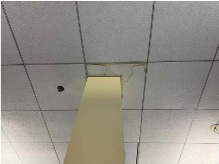
Fig. 39. Water leaks below defective flashing at flat roof above.
