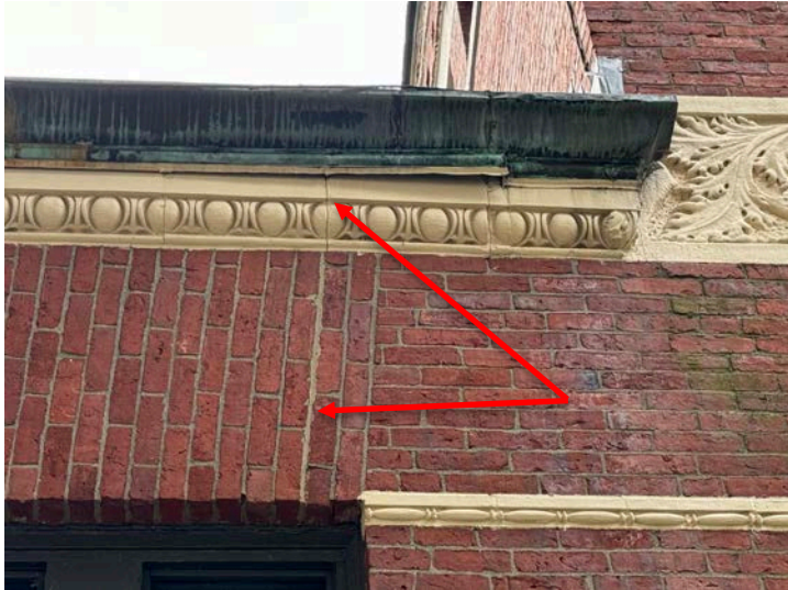
Fig. 1. Step crack through brick joints and sandstone trim.
