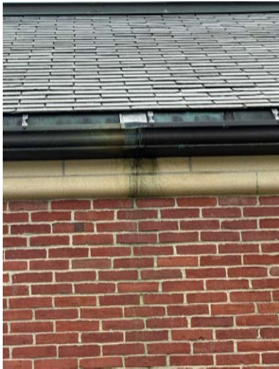
Fig. 37. Open seam on copper gutter causing copper staining below.
