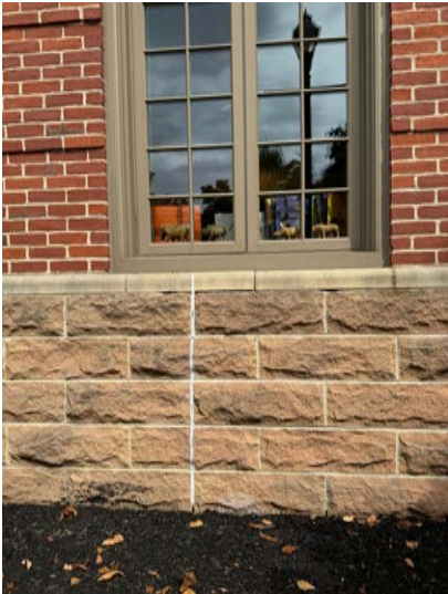
Fig. 31. Sealant material at expansion joints dried and shrinking.
