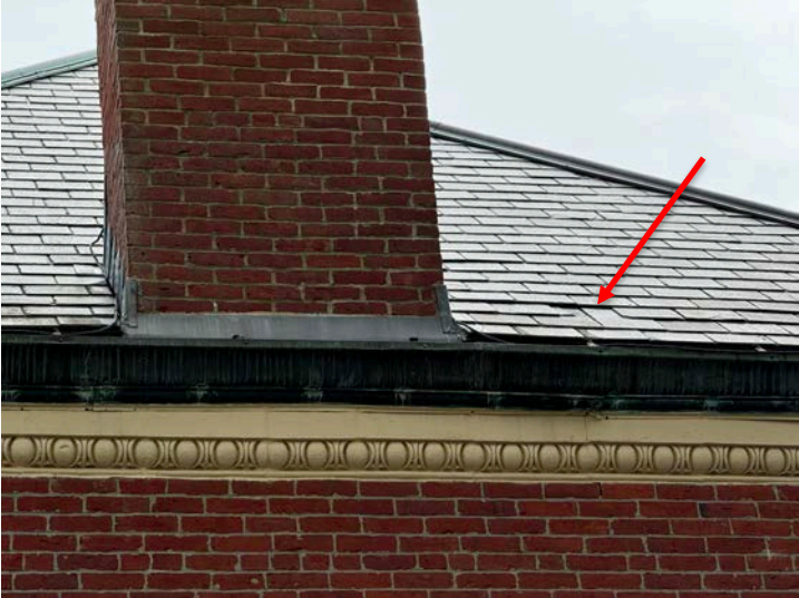
Fig. 9. Slate roof around west chimney showing loose and missing slate.
